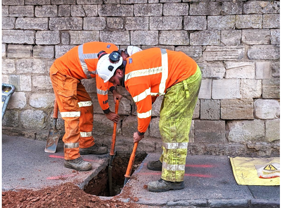
Workmen digging a trial hole on the first evening. Work went on all night to resolve the problem as quickly as possible.
